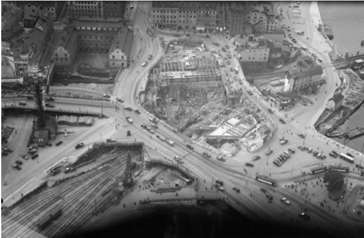
East from above, Slussen during work. Photo: Oscar Bladh, 1932. Stockholm City Museum.
