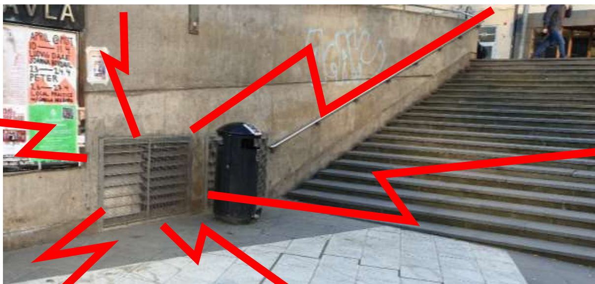
Image 8 – Loud ventilation shaft at Sergels Torg, April 15 th , 08:13, 3,6°C, Sunny
